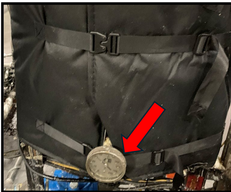
Figure # 16 Day Tank Monitor
