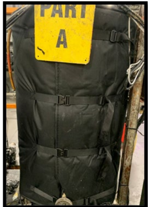
Figure # 15 Day Tank Gravity A and B
